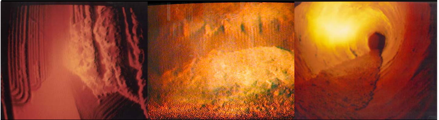
UPPER FURNACE TUBES
