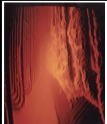
UPPER FURNACE AREA VIEWED WITH SF12IR
